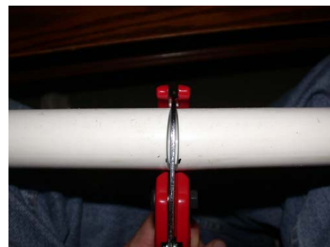
FIGURE 3: CUTTING PVC PIPE. ONCE A LENGTH OF PIPE HAS BEEN MEASURED, A RATCHETED PVC PIPE CUTTER PROVIDES A CLEAN AND EASY METHOD OF CUTTING PIPES. TWO VIEWS OF CUTTING THE PIPE ARE SHOWN IN THE BOTTOM TWO PHOTOS.
